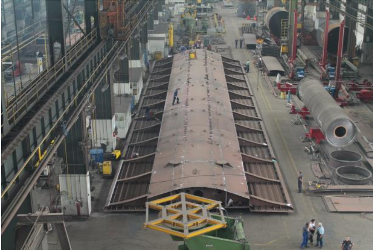
Trial assembly of bridge structure sections for Trogir mainland – Čiovo island bridge (Viadukt d.d.)
